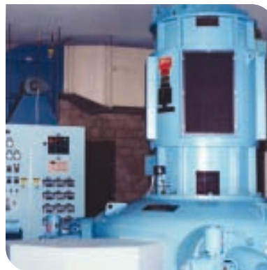
Hydroelectric Power Plant
