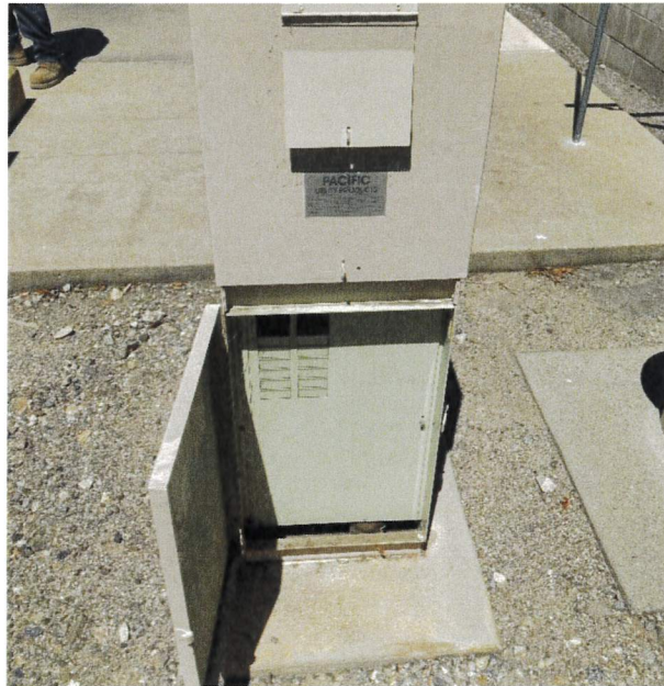
Figure 3.1 – Existing Meter Pedestal Mounted on Concrete Pad
