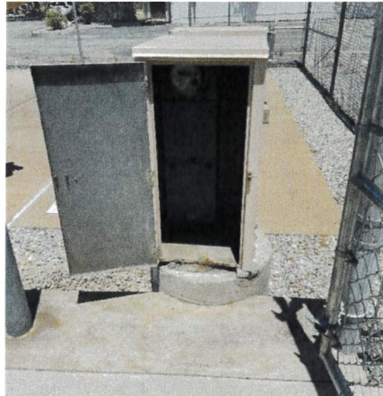
Figure 6.1 – Existing Service Pedestal Mounted on Concrete Block
