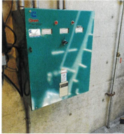
Figure 4.4 – Existing Automatic Transfer Switch to be Replaced.
