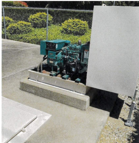
Figure 4.3 – Existing Generator to be Replaced.
