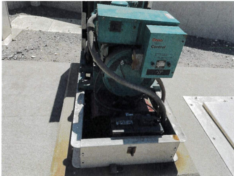
Figure 3.3 – Existing Generator to be Replaced
