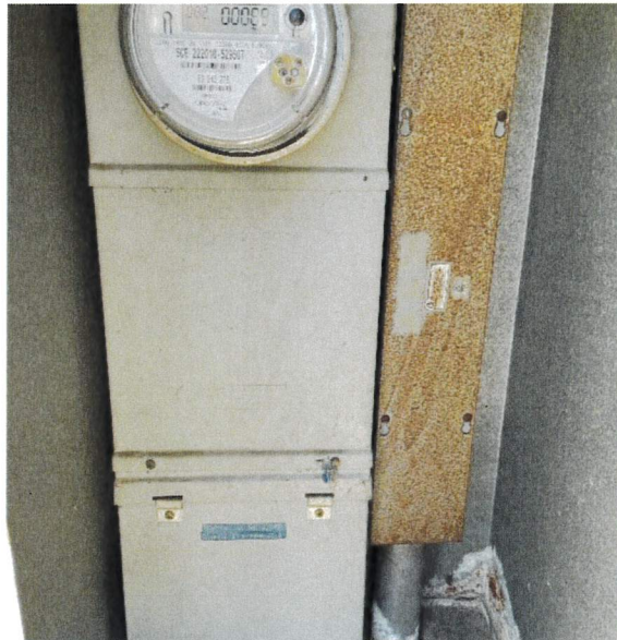
Figure 4.1 – Existing Service Pedestal Mounted on Concrete Pad
