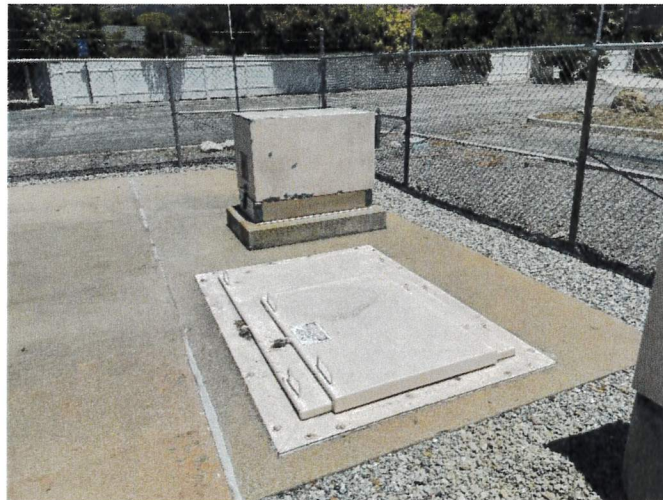
Figure 6.2 – Existing Generator to be Replaced.
