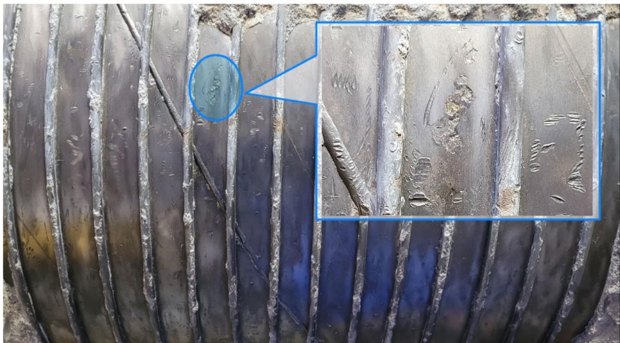
Figure 2 – Observed Area with Localized Pitting in Pipe 940, from PICA’s Report Appendix A (v1.2)
