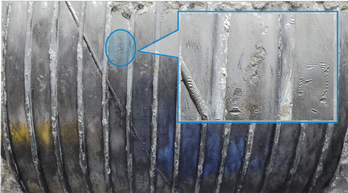
Figure 24. Pipe 940 was excavated on May 8, 2024, to allow for further validation of the reported defect. Note that the Dec 13 UT validation identified an OD defect at the same location, which corresponded to the localized wall loss signal in the RFT data. Both the steel cylinder and bars were found to be in excellent condition with no apparent corrosion. However, a cluster of shallow pits were observed at the location of the defect identified by both the RFT inspection data and UT validation. The overall area of the pitting cluster measured 0.5" x 1.0" with a UT-measured depth of ~68% RW.
