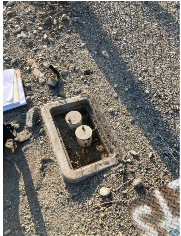
Schedule III – Isolation ETS at Freeway 210 Bridge
