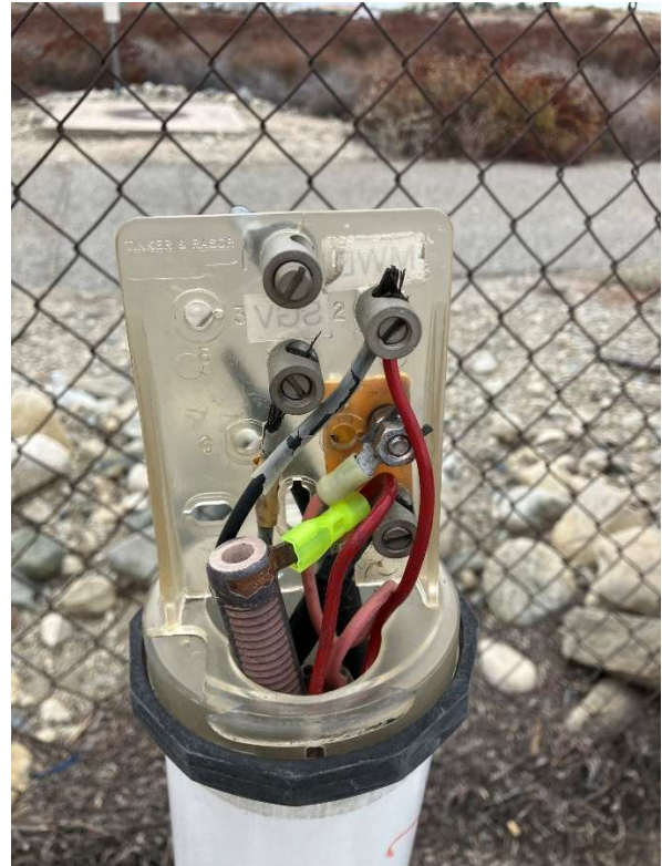
Schedule V – Sta. 1683+50 Bonding Test Station
