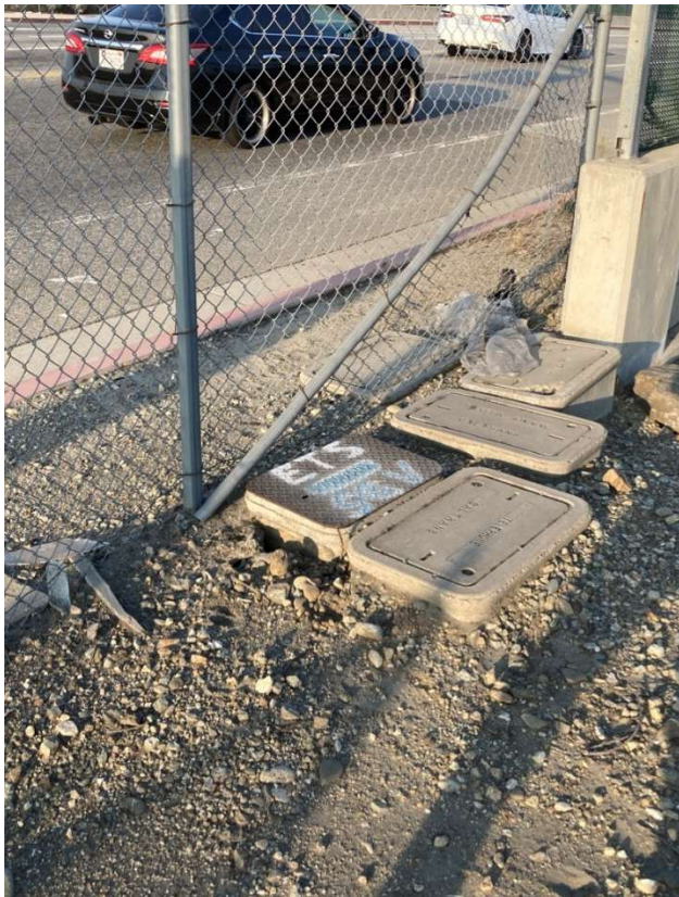
Schedule III – Isolation ETS at Freeway 210 Bridge
