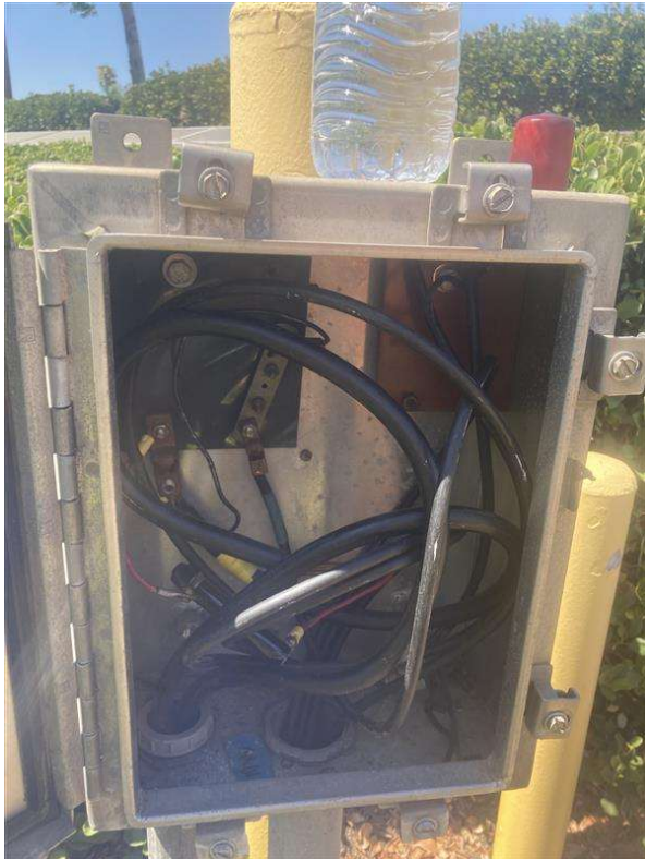
Schedule V – Sta. 1364+00 Bonding Test Station
