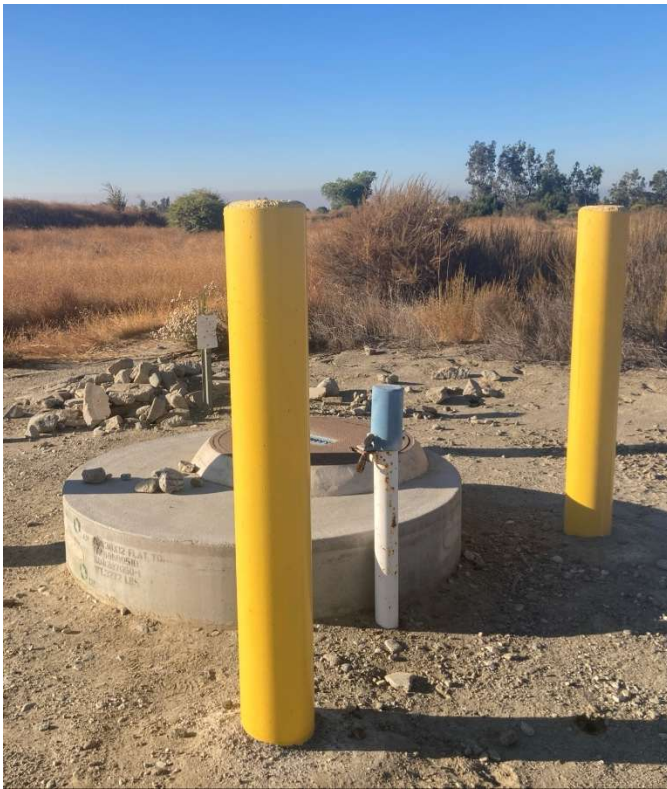
Schedule VI – Sta. 1764+00 Bonding Test Station
